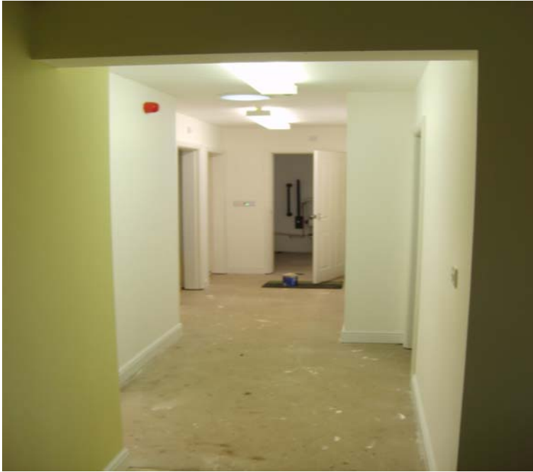
The Corridor leading from the main room to the toilets. 25% of painting to do + 2 doors to hang to complete this area
